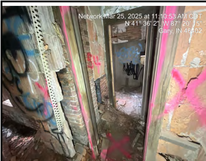
FS-54 Bathroom Completely inaccessible Structural Damage
