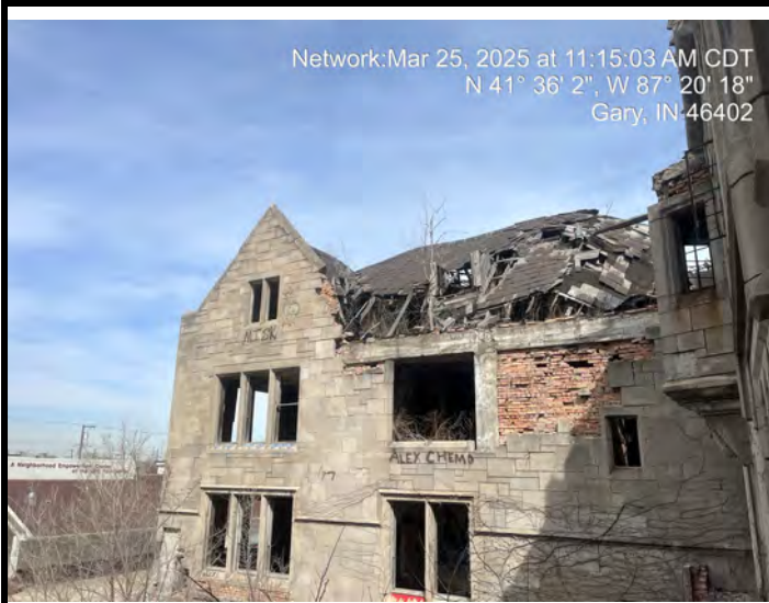
EA-5 Roof Completely inaccessible Structural Damage
