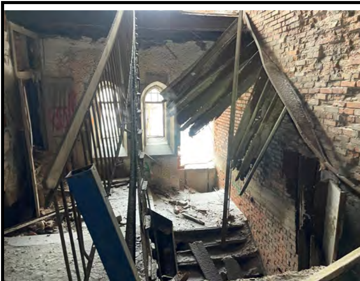
FS-58 4th Floor Completely inaccessible Structural Damage
