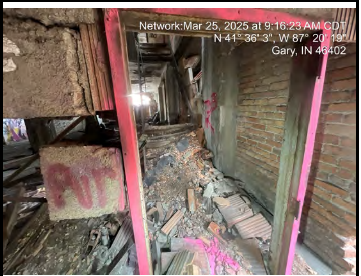
FS-33 Staircase Completely inaccessible Structural Damage
