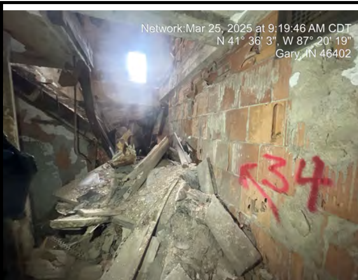
FS-34 Staircase Completely inaccessible Structural Damage
