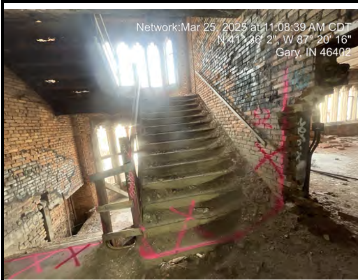
FS-52 Staircase Completely inaccessible Structural Damage
