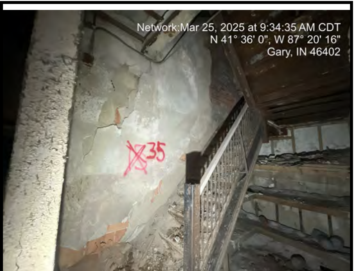
FS-35 Staircase Partially inaccessible
