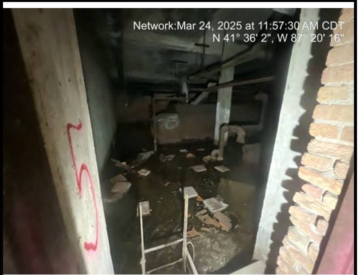
FS-5 Boiler room Completely inaccessible Water Damage
