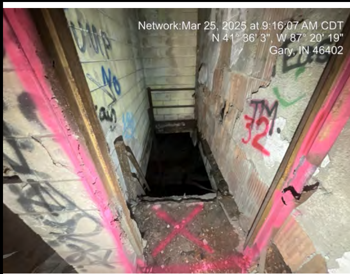
FS-32 Staircase Completely inaccessible Structural Damage
