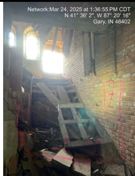
FS-17 Staircase Completely inaccessible Structural Damage
