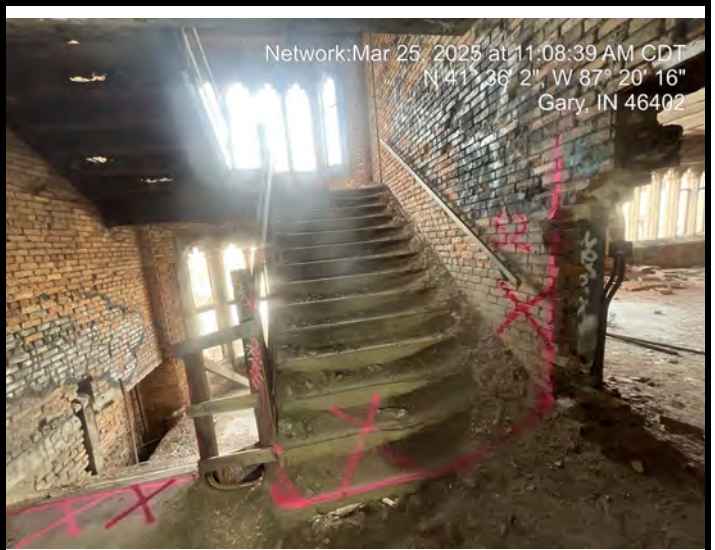
FS-57 3rd Floor Completely inaccessible Structural Damage
